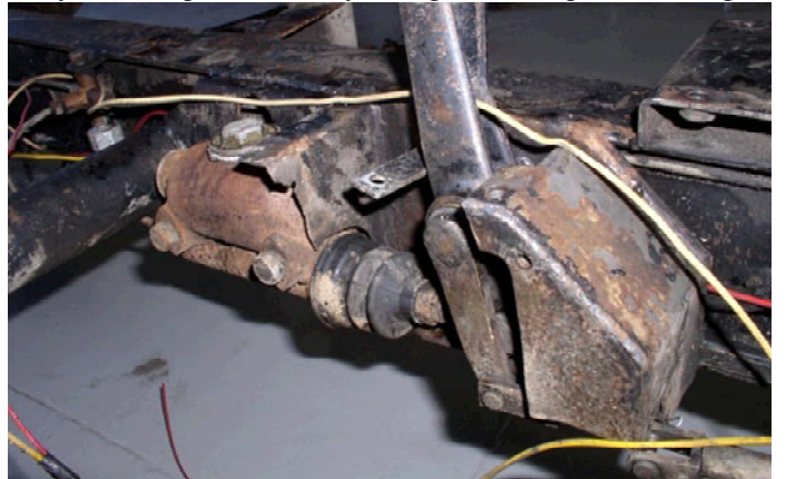
Fig.2 The remains of a pedal box that has been butchered during a previous "repair".
